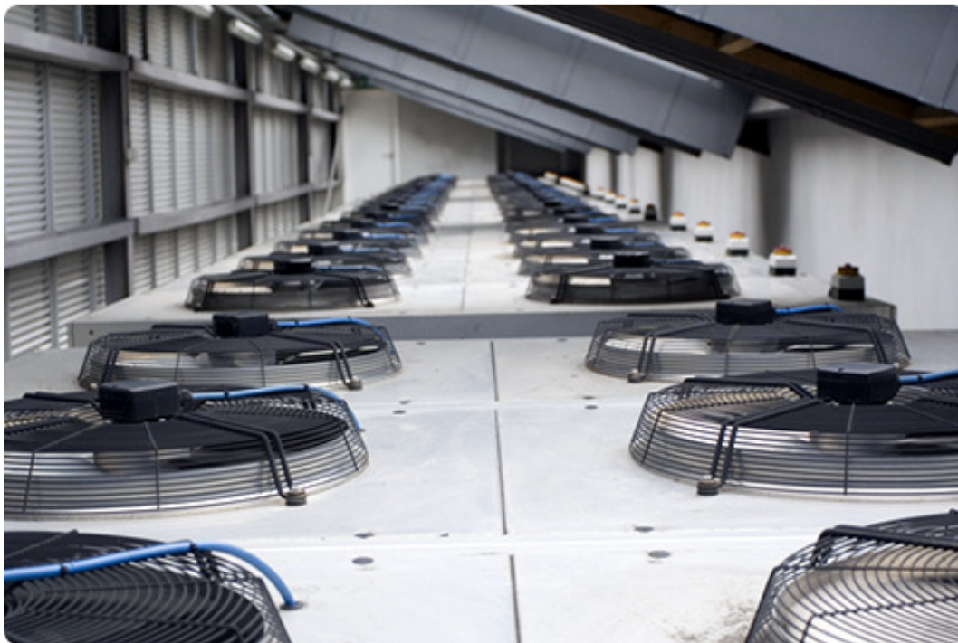
Banks of extractor fans pull warm air from the top of cabinets
