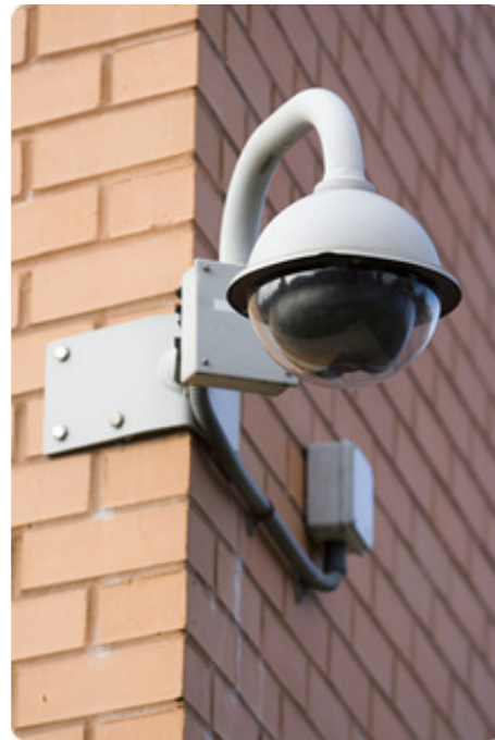
External CCTV coverage
